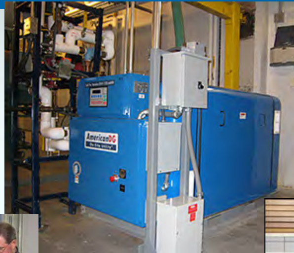
Apartment Building 75kW e
